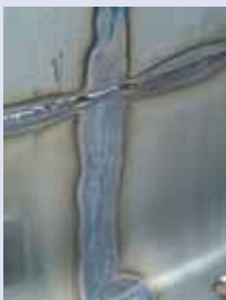
Bluish heat tinting around welds in a 4301 stainless steel tank. If kept untreated, the risk of pitting corrosion in the bluish zone is significant, and therefore, the heat tinting must be removed. The easiest way to do this is a pickling.
